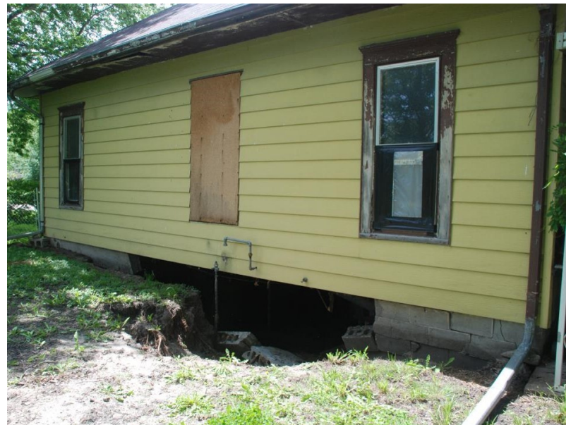
A potentially substantially damaged house
